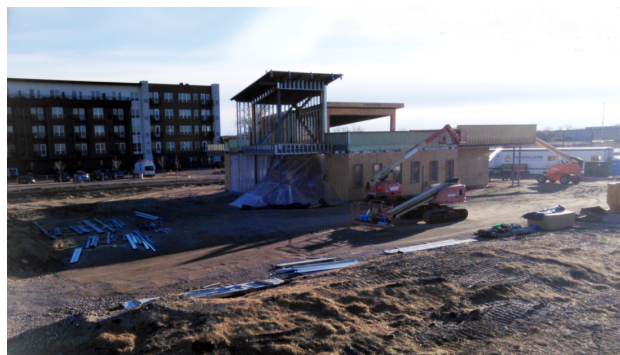
Future location of our Blaine office on March 13, 2026. View the construction camera online at idealcu.com/blaine-construction
